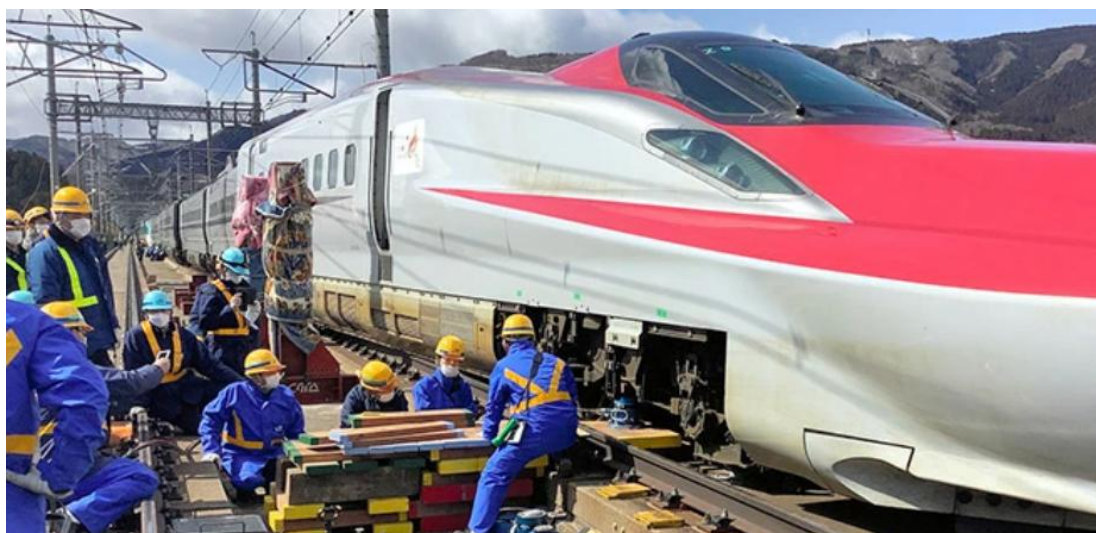
Workers begin installing hydraulic jacks to lift the carriages of the Tohoku Shinkansen bullet train that derailed as a result of an earthquake, in order to resume services before Golden Week. Source: East Japan Railway Co., March 2022.
